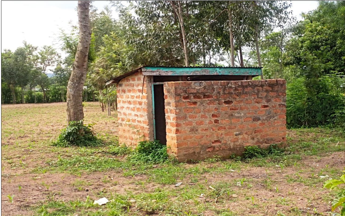
3. Dilapidated latrines at Omoloi Primary school
