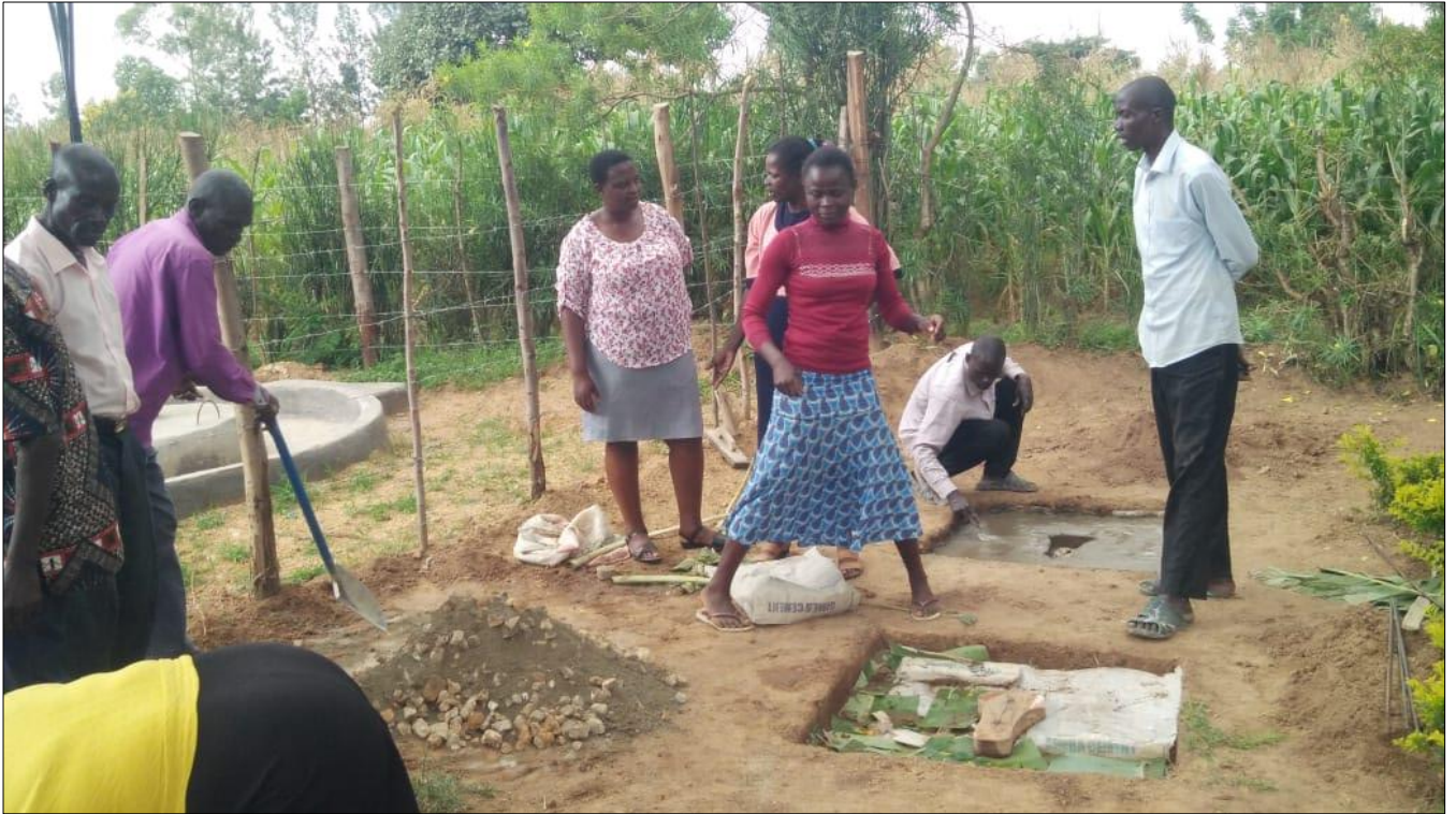
11.0 Community members at Imani Bora site making SANPLAT slabs at their water point site.
