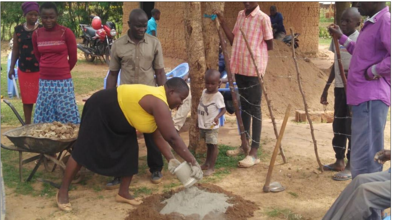
12.0 Women participating in preparing concrete mix for SANPLAT Slabs casting for Ecological Sanitation latrines
