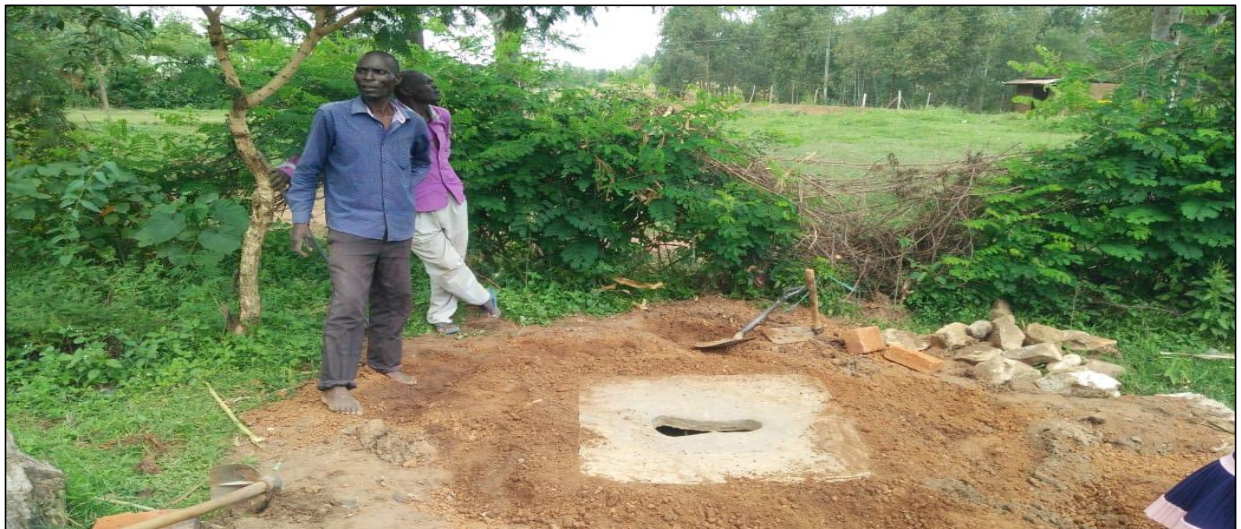
8.0 Mounting of SAN PLAT slabs ready for latrine construction at Imani Bora Village
