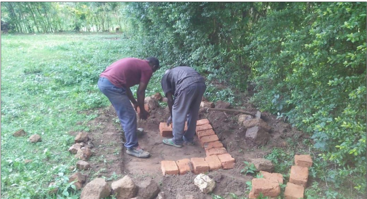
10.0 Demonstrating how to prepare the foundation wall for SAN PLAT slab mounting & latrines construction in Sinoko village for Bititi Youth Group members
