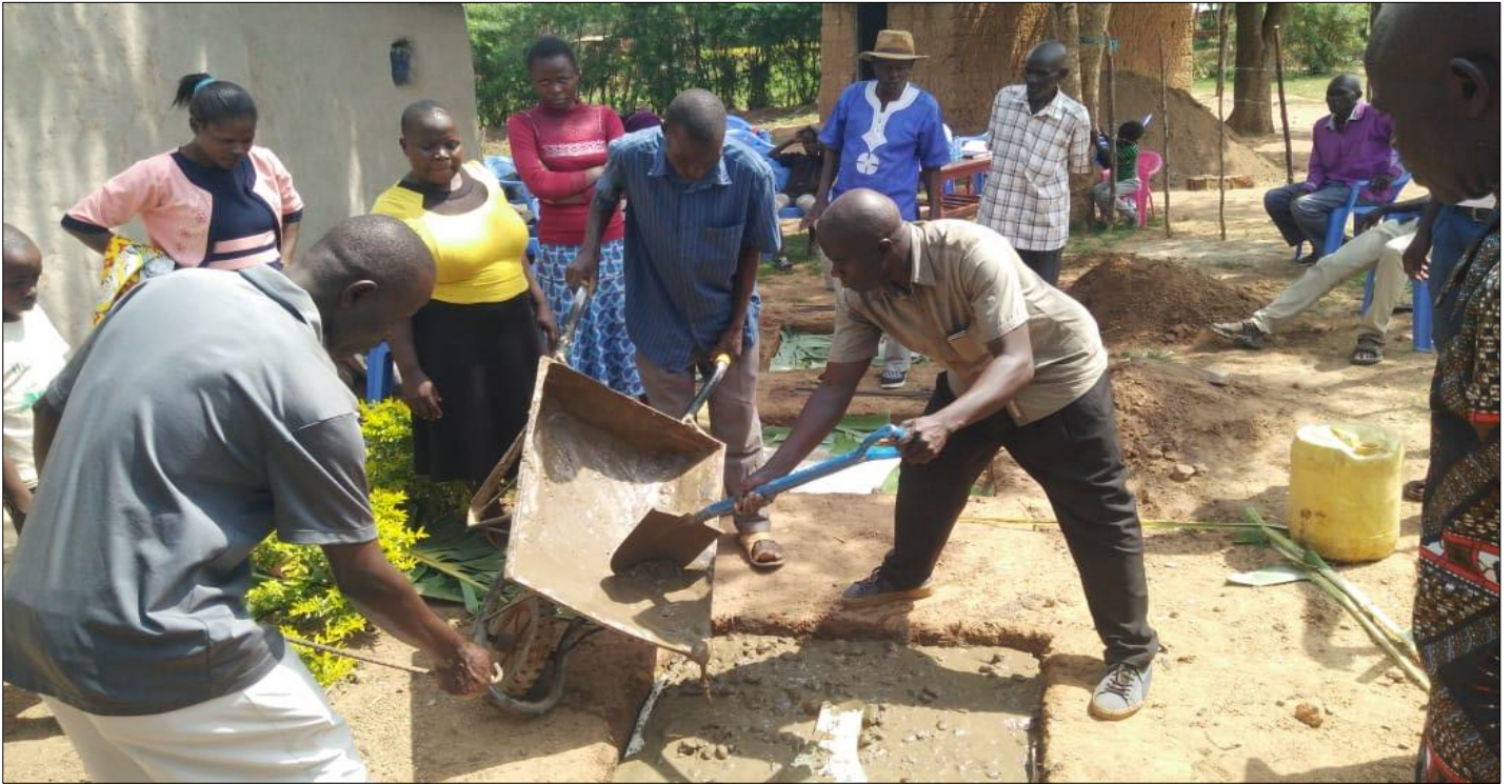
13.0 Community participation in development of households SANPLAT slabs for Ecological Sanitation latrines at Imani Bora water point site
