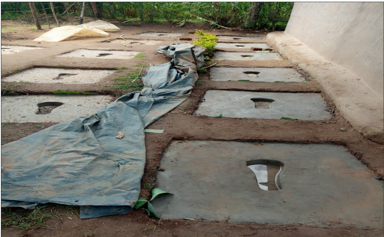
14. SANPLAT slabs manufactured by community members of Imani Bora water point being cured ready for latrines construction at households' level.
