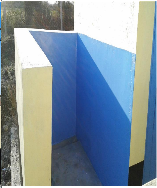
10. URINAL FOR THE BOYS VIP LATRINES
