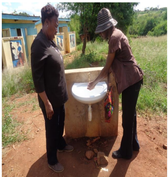
Water installation at the school next to the washrooms
