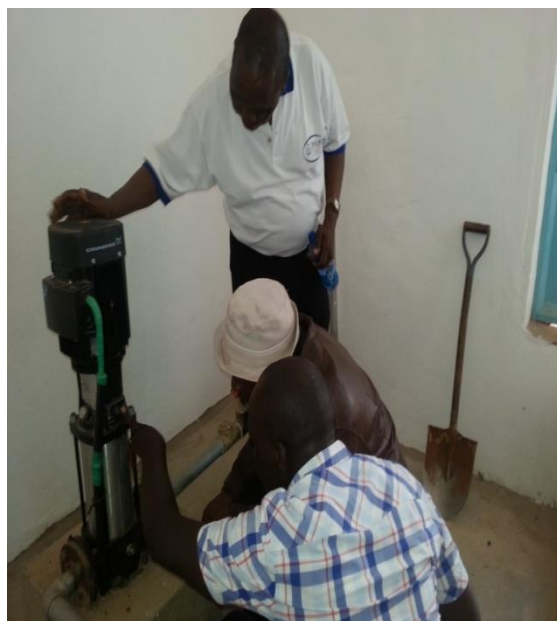
Inside the Pump House at the intake
