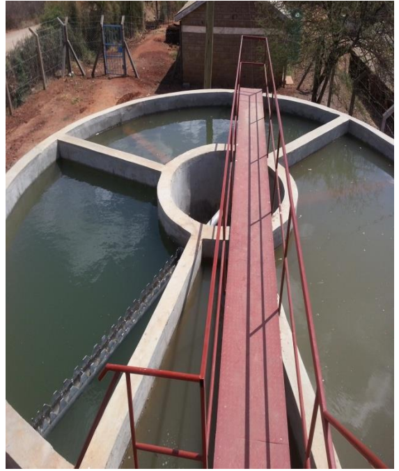
Top of the coagulation tank
