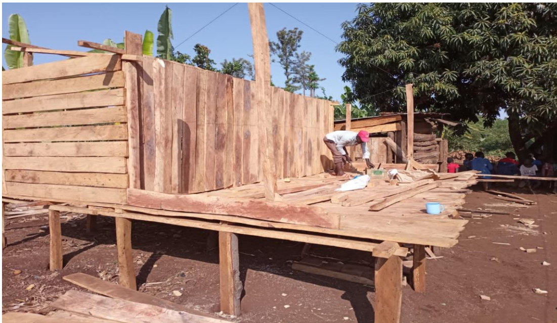
11. Group members of Wendo Mweiga women group constructing their animal pens/shades in preparation of the Dairy goats to be received from the project
