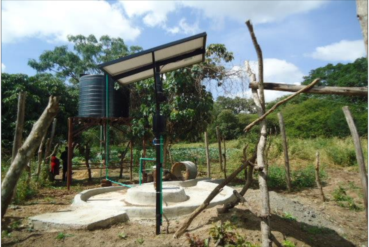
7.0 Sykoka water point with solar pumping system and raised storage tank-drip irrigation at edge of the water point
