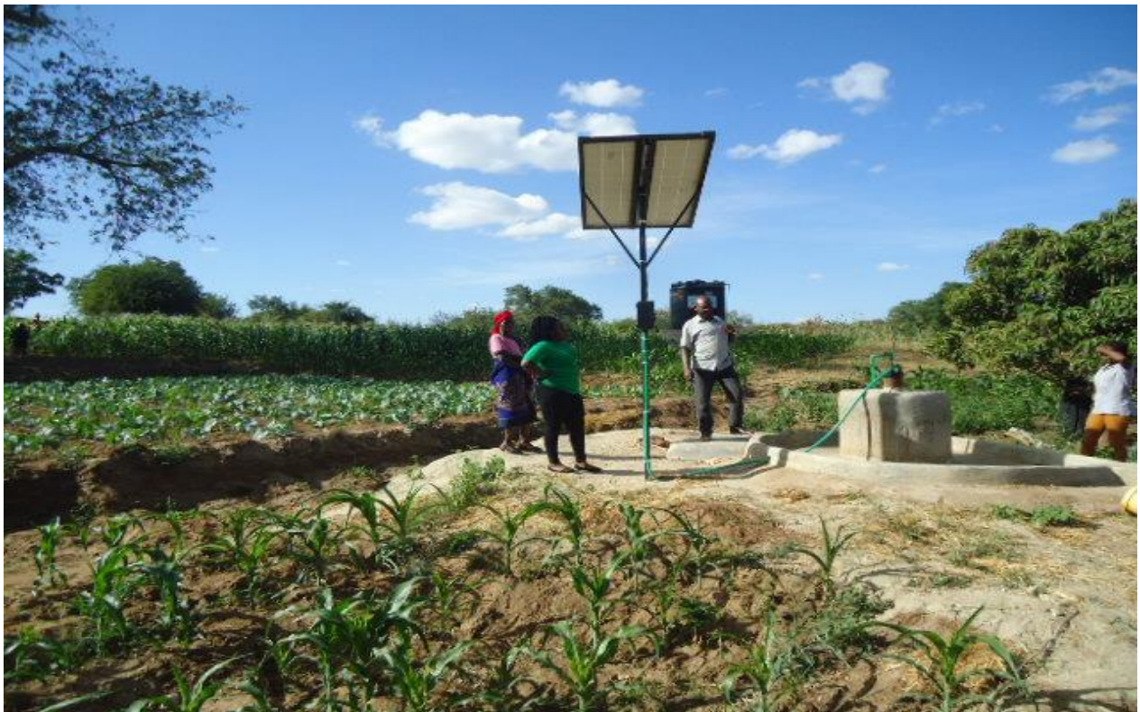
6.0 Kyeni Chan Ngini water point with solar pumping system and drip irrigation farm
