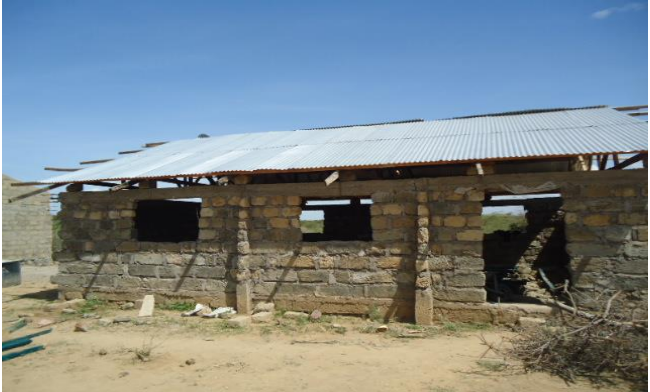
1. Loruk Day Secondary school building nearing completion –reconstruction supported by the project
