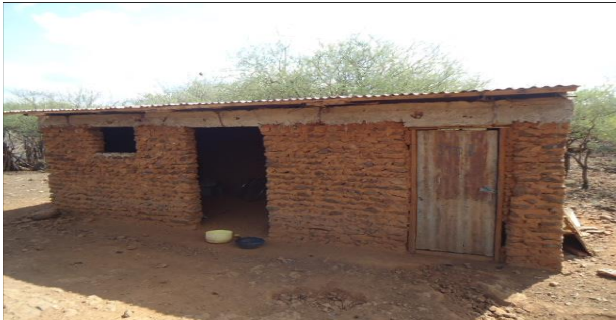
10. A house reconstructed with project for vulnerable household nearing completion in area around Lake Baringo-Ngenyin village
