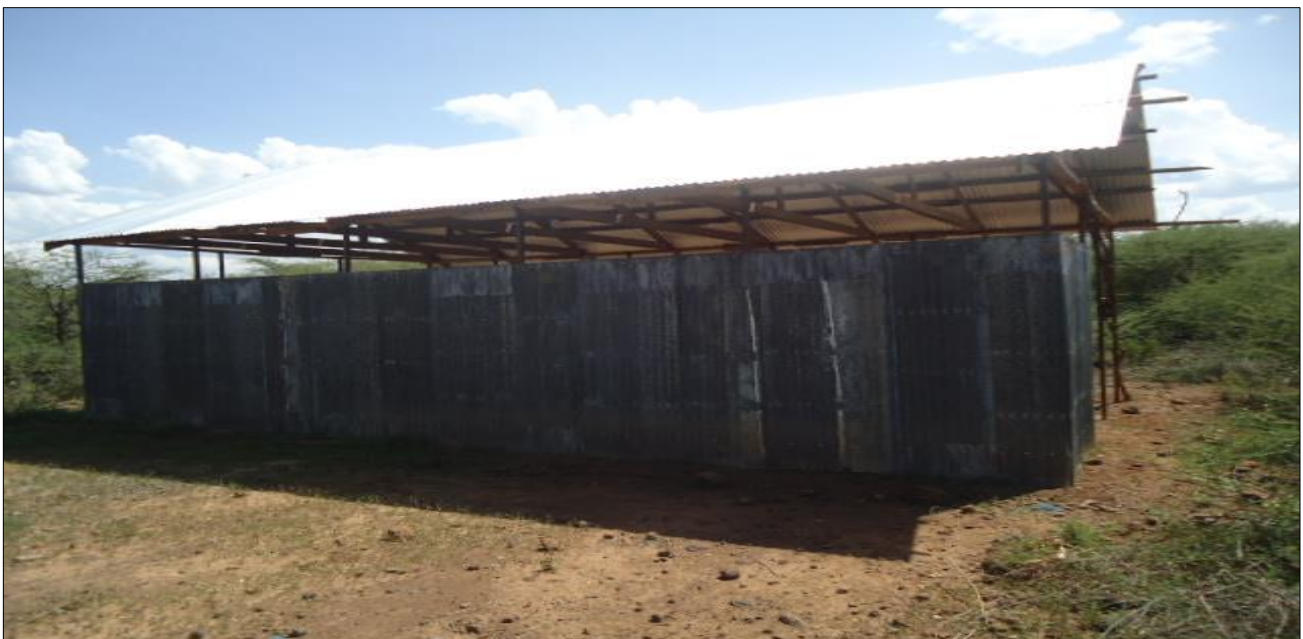
8. Chelelyo ECD Center reconstructed by the Project school relocated due to floods
