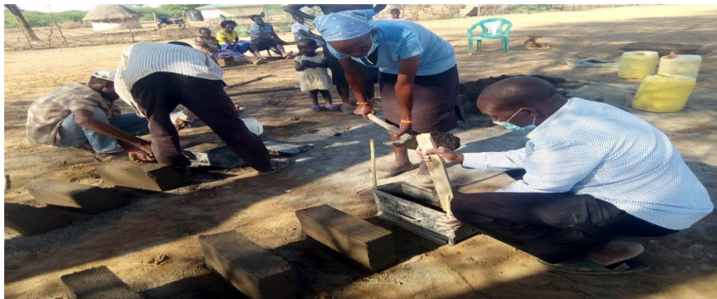
5. Preparing & manufacture of trapezoidal blocks for SANPLAT latrines lining for weak soil formation/flooded areas
