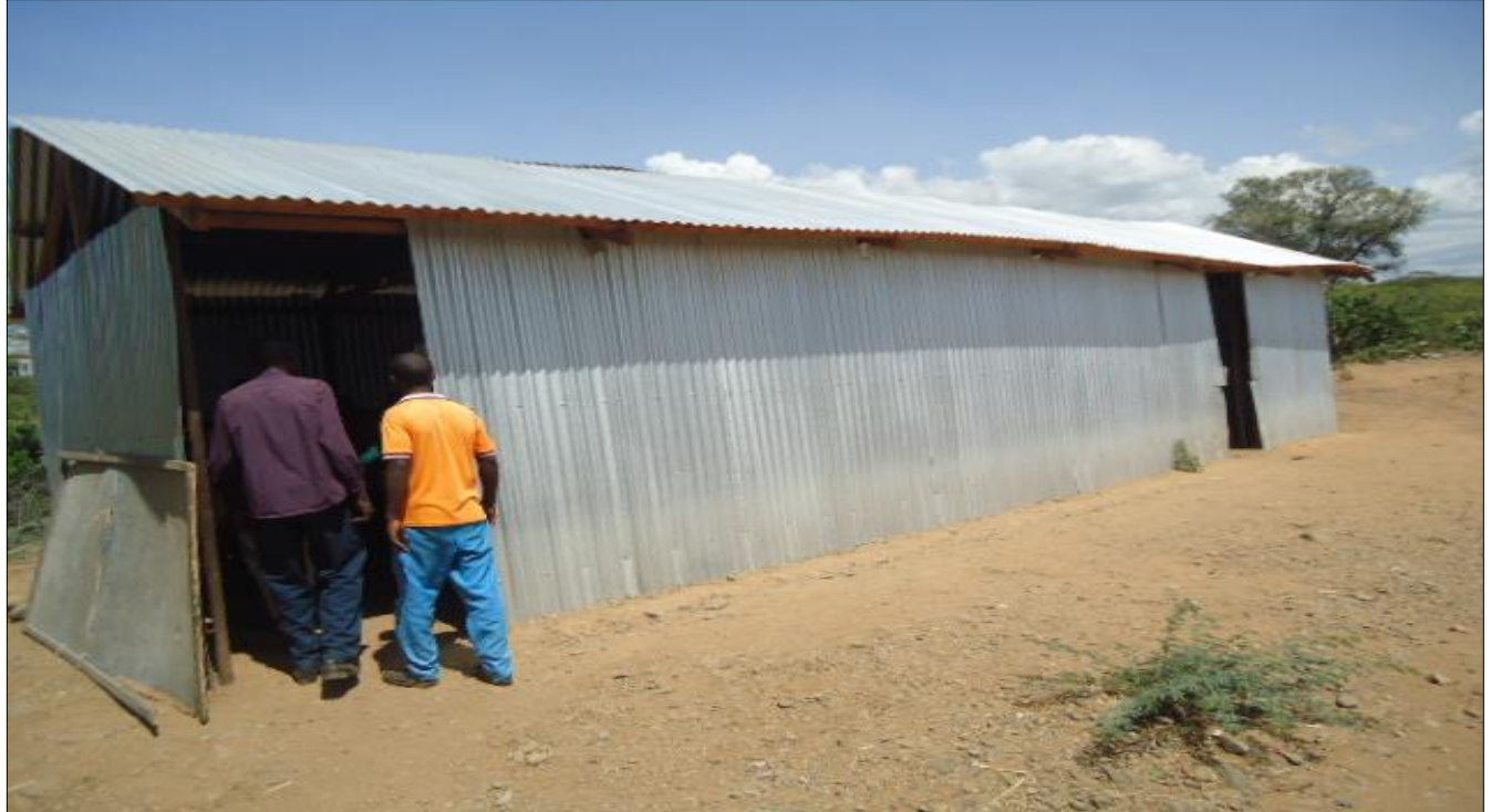
3. Ngambo Primary School classroom reconstructed after school relocation due to Lake Baringo floods
