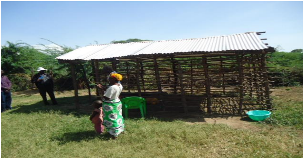
11. A vulnerable household Ms. Grace Lonoo relocated due to floods with their house under construction with support from the project in Lospeken area of Eldume village
