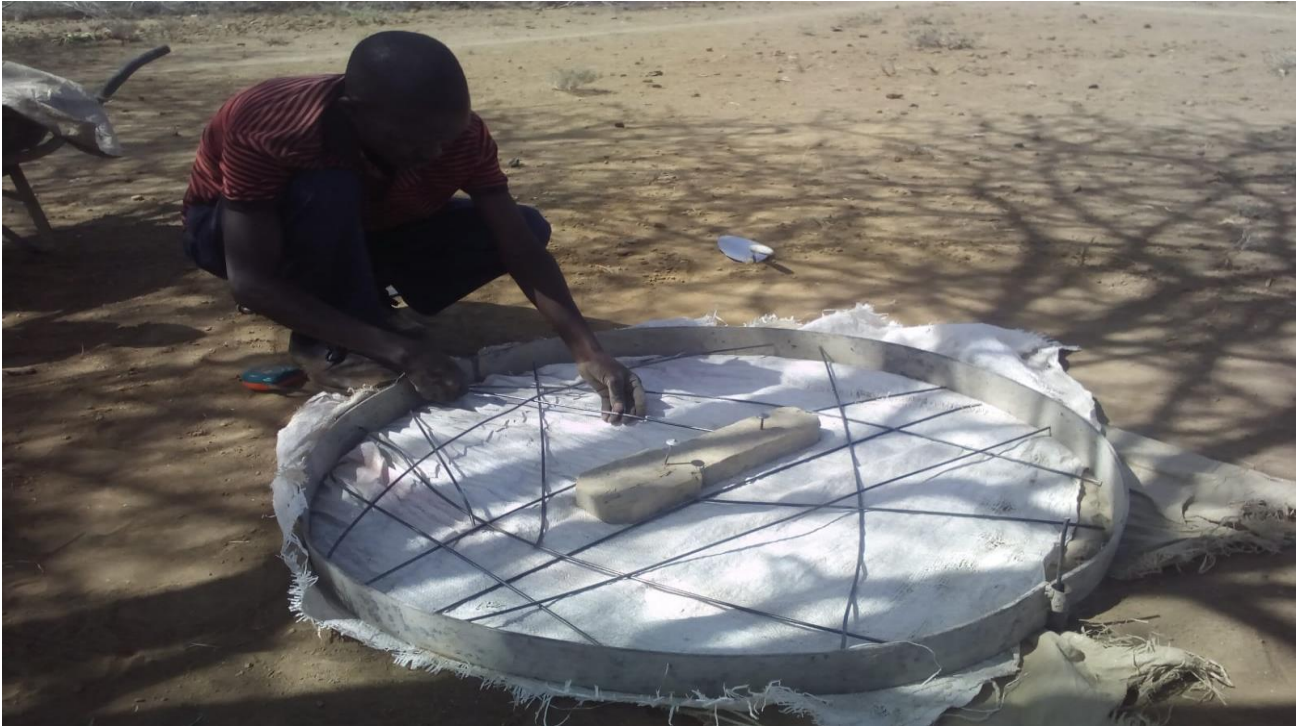
1. SANPLAT Latrine slab being constructed for improved sanitation in relocated village for vulnerable villagers displaced by Lake Baringo floods
