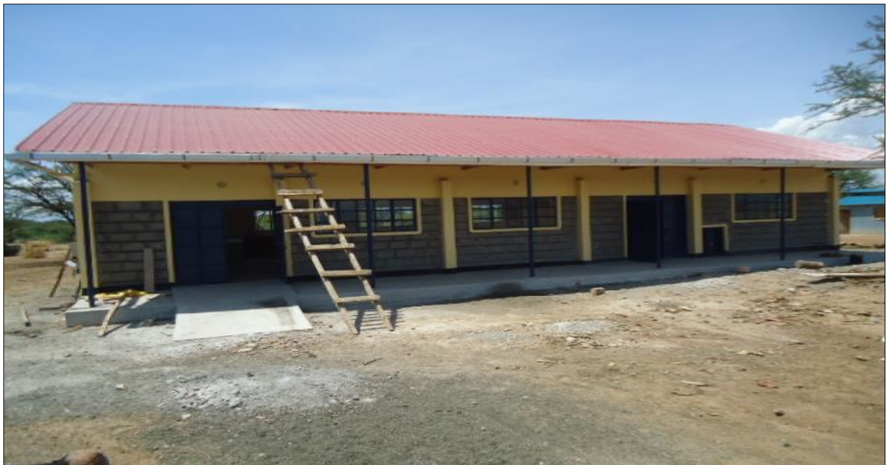
2. Ngambo Girls School laboratory being completed –Reconstruction supported by the project after relocation
