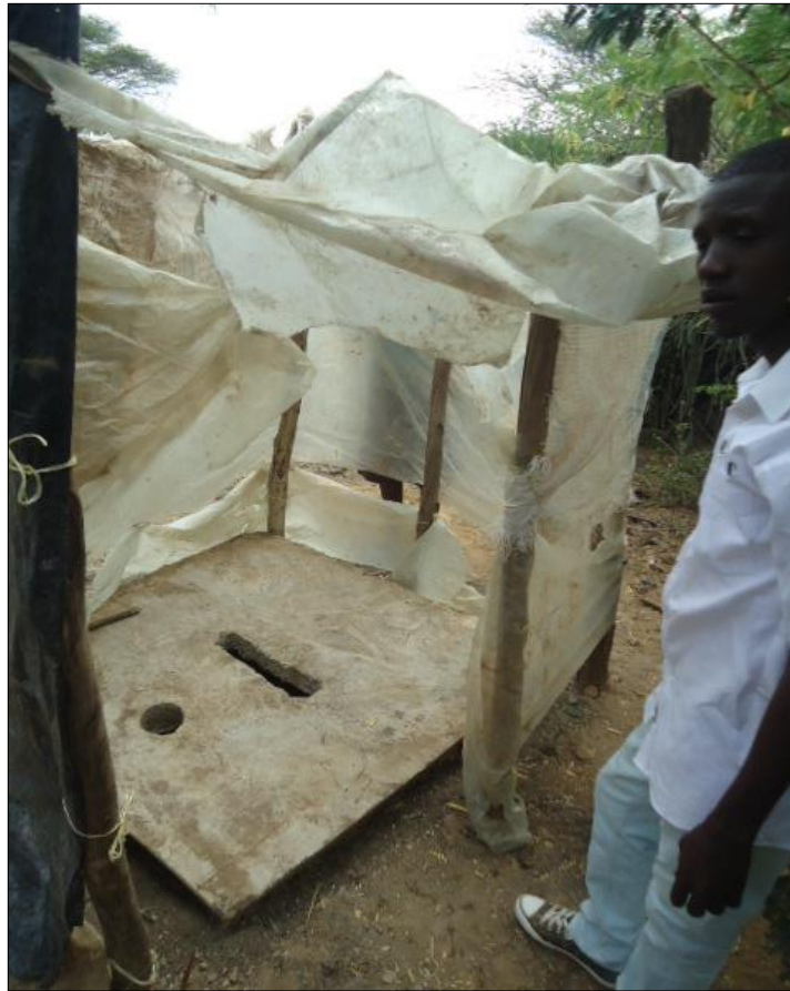
10. Temporary structure household latrine in use with SANPLAT slab in Kabikok village
